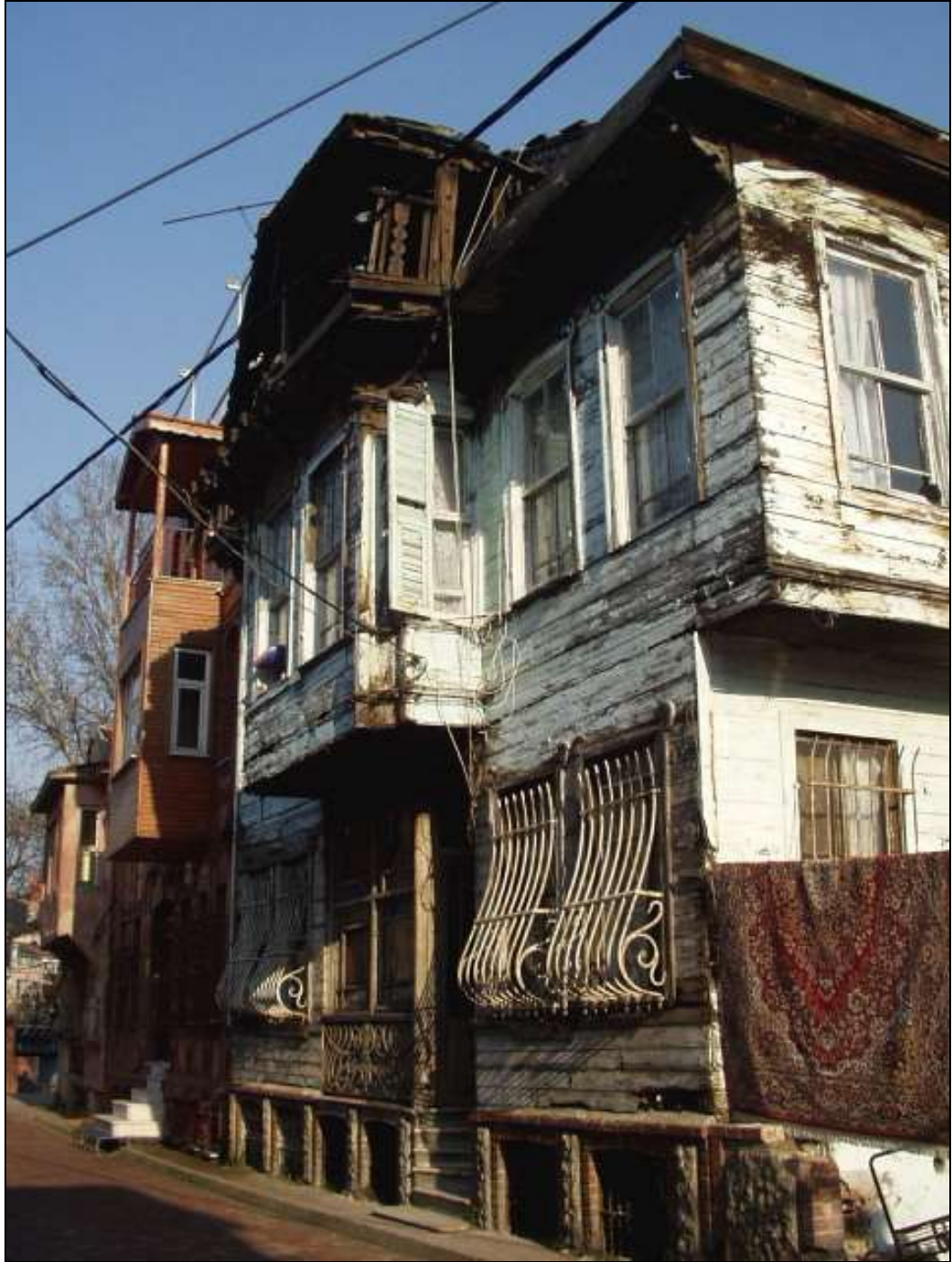
Figure 27. Building in Bad Condition
