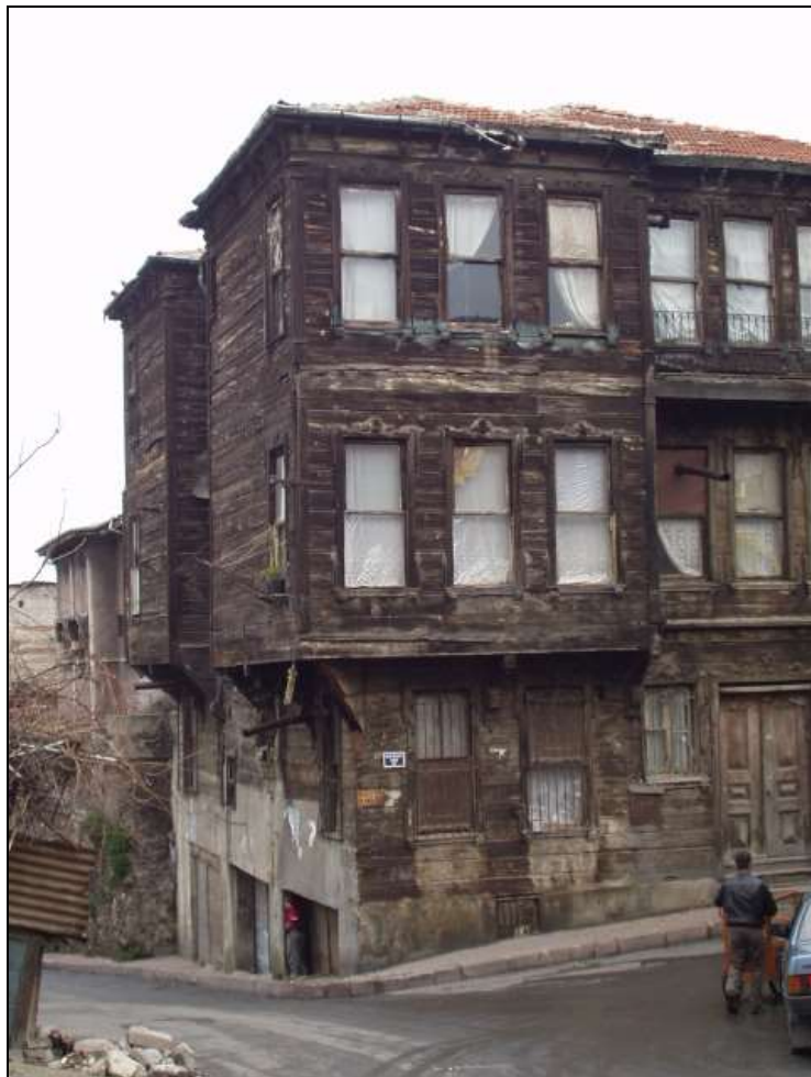
Figure 71. A Ruined Listed Building
